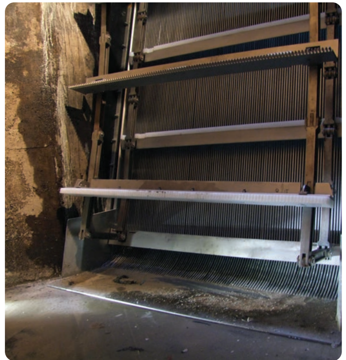
Curved Bar Rack at Channel Bottom
